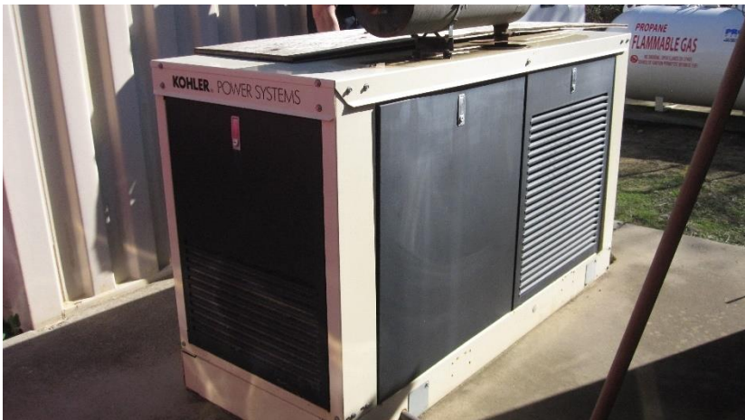
Photograph 7. View of the emergency generator (with associated propane AST in the background) in the southwestern portion of the subject property, facing south.
