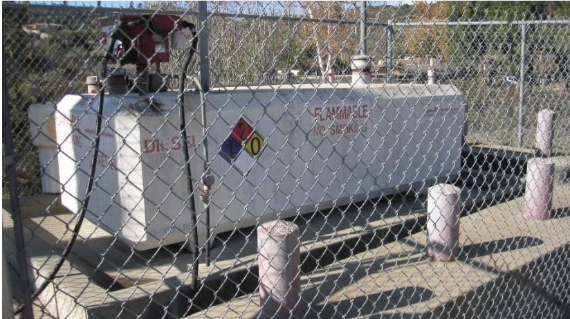
Photograph 5. View of the diesel AST in the northwestern portion of the subject property, facing northwest.
